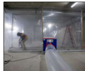
Worker drilling concrete inside an enclosure equipped with a "negative air" unit
