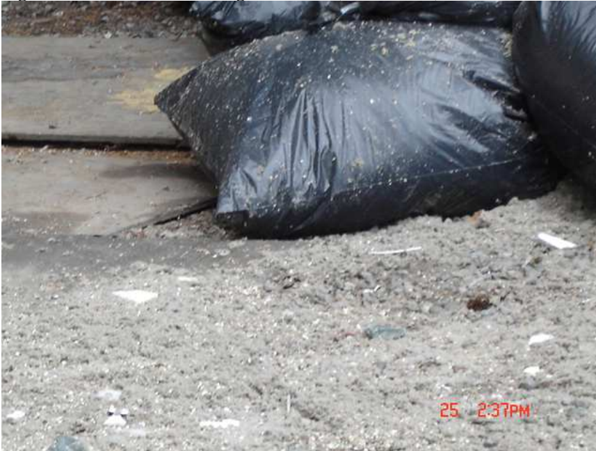
Figure 2 - Asbestos Containing Insulation (Vermiculite)
