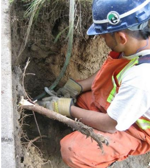
Figure 3: Ops III worker cutting ¾" copper service pipe with a pipe cutting tool.
