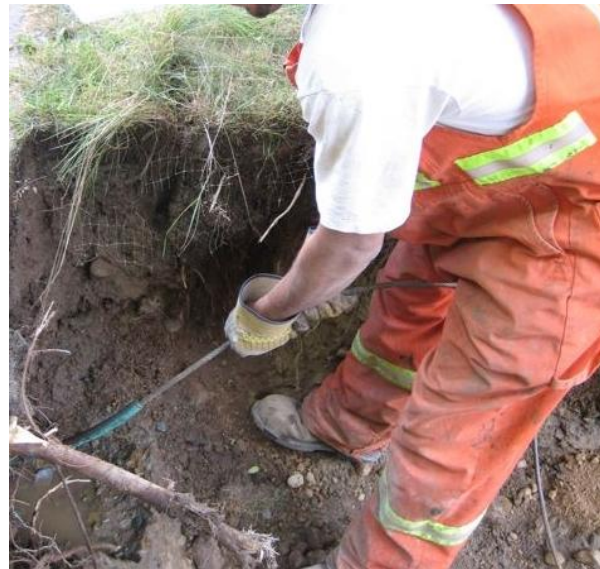
Figure 4: Ops III worker feeding cable through the existing pipe to perform a renewal of service.
