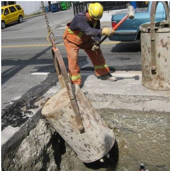
Figure 9: Ops III worker hammering drum to release residual cement on a fireline job.
