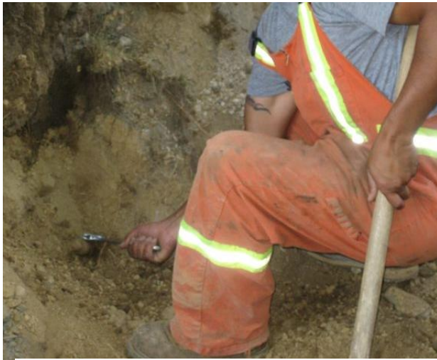
Figure 1: Ops III worker turning off service at the main with a wrench.
