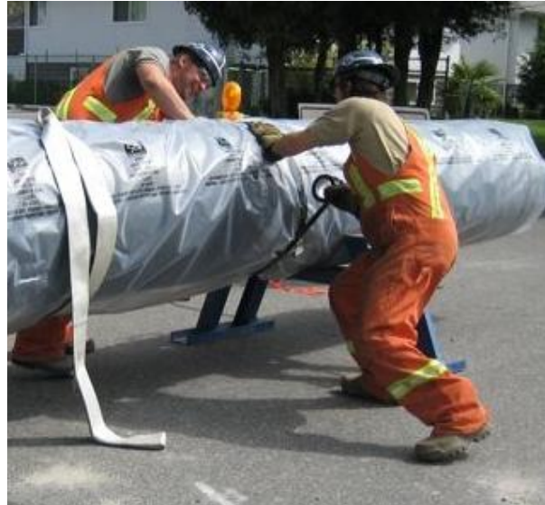
Figure 6: File photo of Ops III workers wrapping pipe, (this is larger diameter than firelines pipe).
