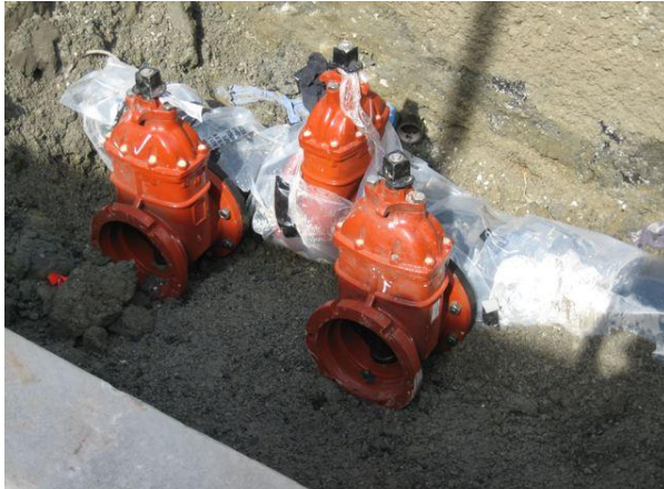
Figure 5: Valves in place that were assembled above ground by Ops III workers.
