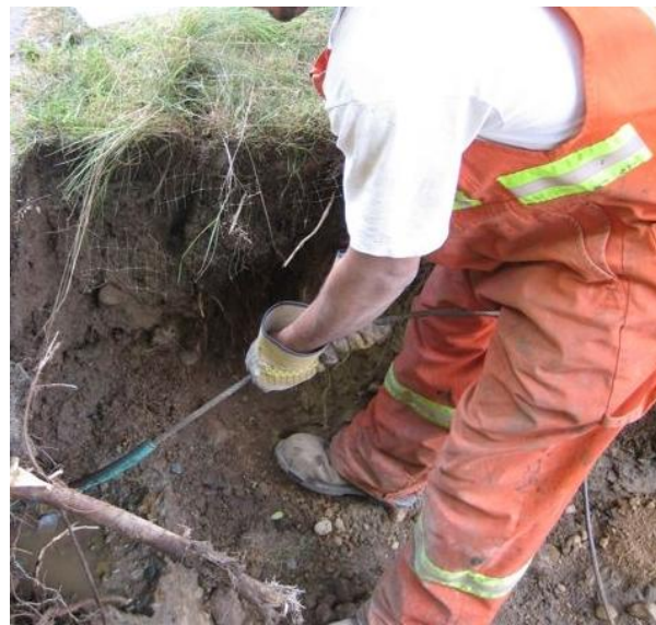
Figure 4: Ops III worker feeding cable through the ¾” pipe to perform a renewal of service.
