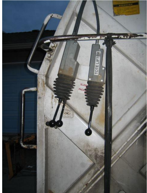
Fig 6: Tote lift & hopper control levers.
