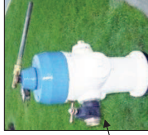
Using hydrant key to open / close hydrant
