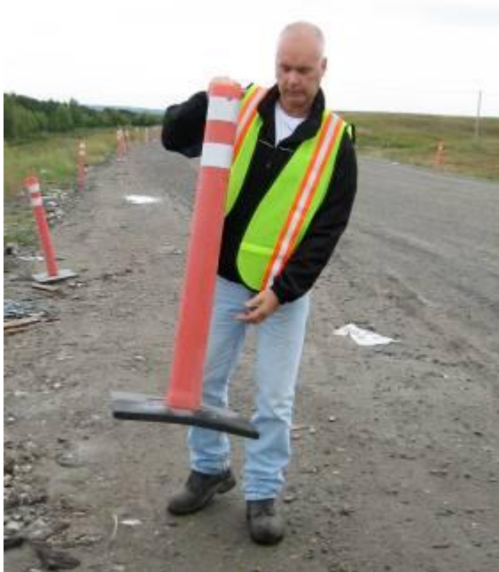
Fig 6: Ops II worker setting up cones to indicate road to main dump.
