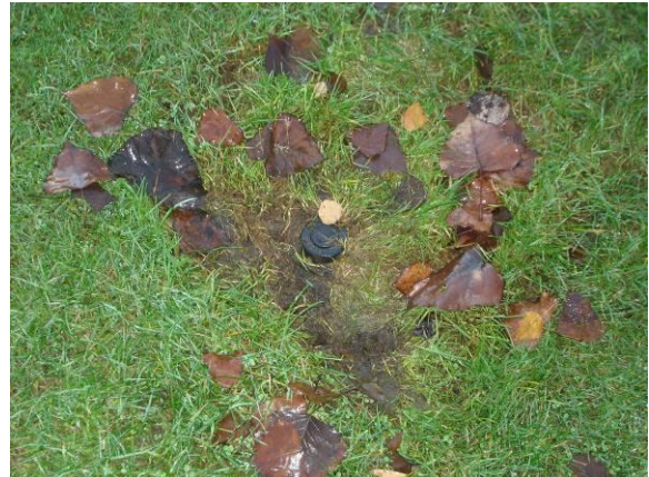
Figure 3: Example of hole around irrigation head.
